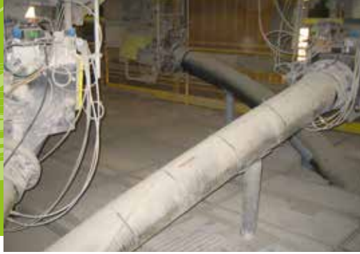
Cement plant 10» Scirocco II for truck loading.
