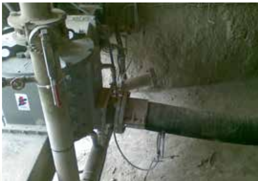
Cement plant Scirocco II hose connected to an airslide.
